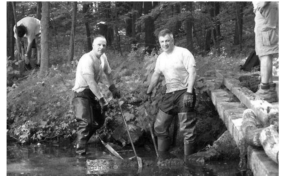
Members of the dam crew hauling debris that was blocking water flow under the dam bridge.
